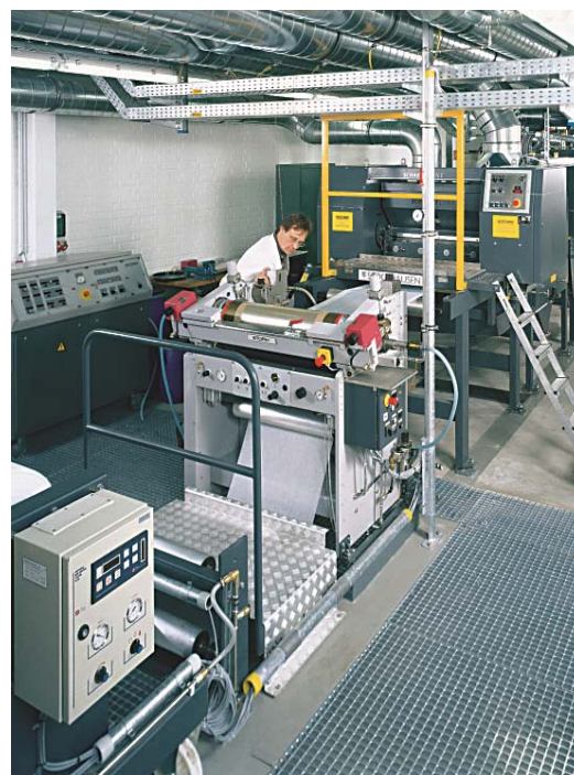
Bozzetto Coating pilote plant in Krefeld, Germany
